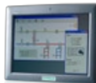
With Regin Panel PC connected to Corrigo Web, the installation can be handled directly on site
